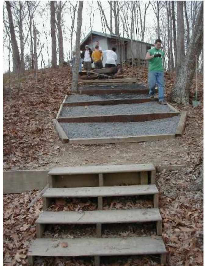
Boy Scout Troop 91 and Sea Scout Ship 91 Work on the path from the Shelter to the Bath House For William King's Eagle Project under Under the supervision of P/R/C John J. Rodgers, SN-CN
